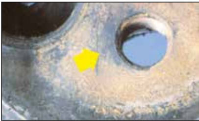
Figure 2 - damaged core refund Bottom deck crack
