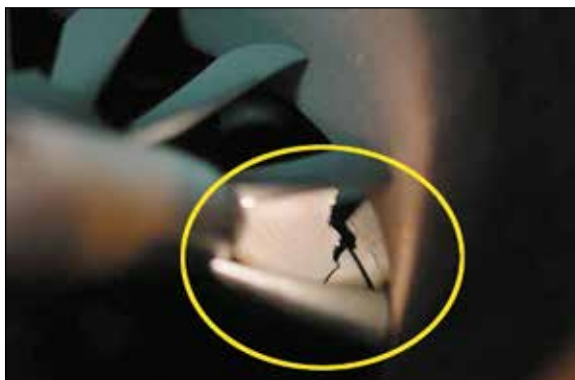
Figure 8 - damaged core refund Hot wheel broken
