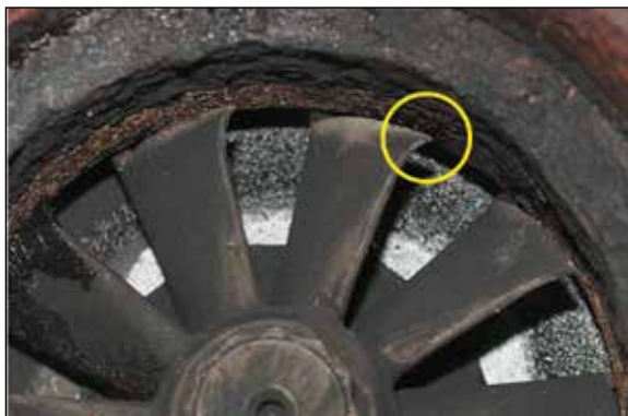
Figure 6 - damaged core refund Hot wheel bent
