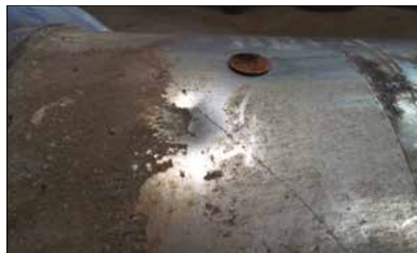
Figure 5 - damaged core refund Non-operational damage - case damage
