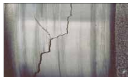
Figure 1 - no core refund Visible crack
